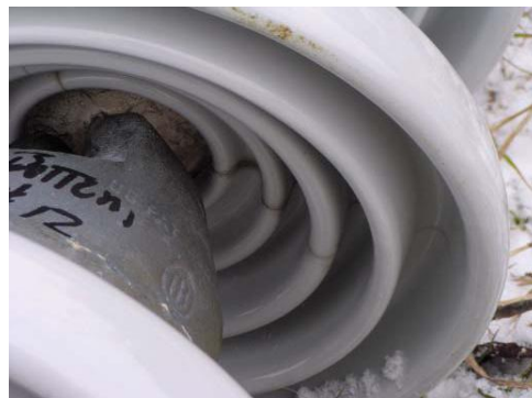
Figure 32: Cracked insulator skirt.
