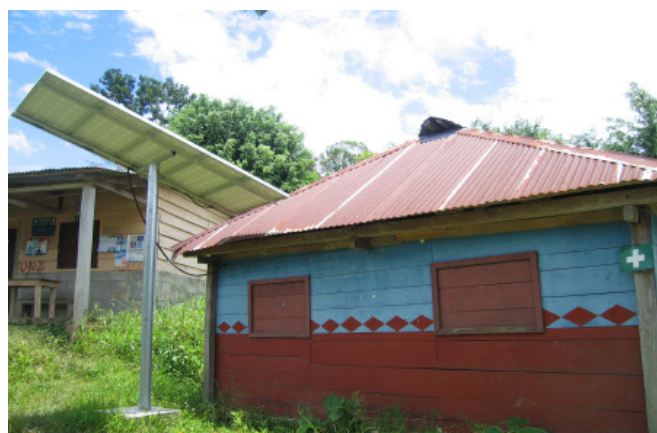
Figure 31: Solar panels in a sanitary center in Copaláa la Esperanza. Source: Energías sin Fronteras, 2009
