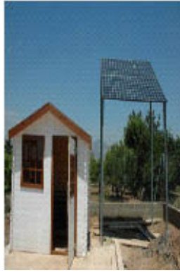
Figure 22. Solar panel connected to a medical post. Source: EsF.
