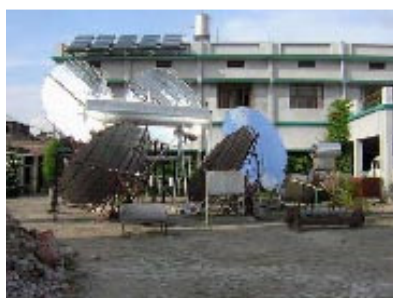
Figure 19. Installation at Patna Solar Center. Source: EsF
