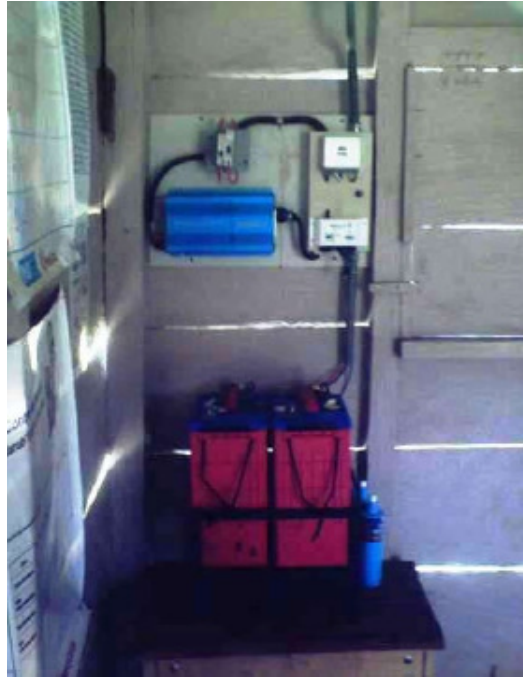
Figure 32: Components of a photovoltaic system in a sanitary center in Sta. Elena Satolohox. Source: Energía sin Fronteras, 2009
