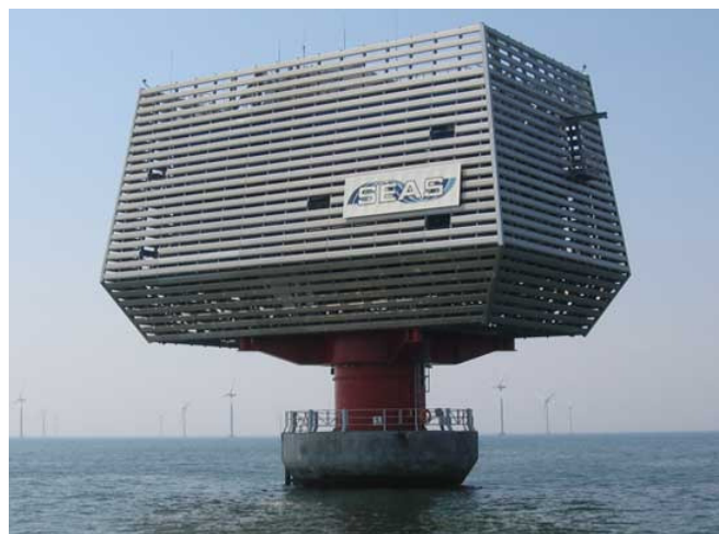
Figure 3.8. Nysted's offshore substations
